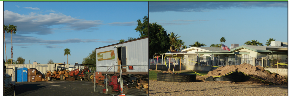
Above: Construction equipment and job trailer fill the west side of the Willowcreek/Willowbrook parking area as work begins on the course.
